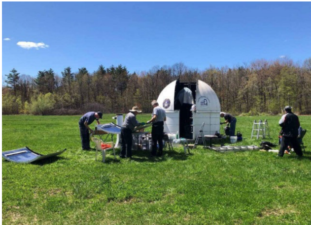
Summer maintenance by the Dome Crew, lead by Observatory Director Alex Stefanescu, included a revamp of the dome shutter mechanism.
