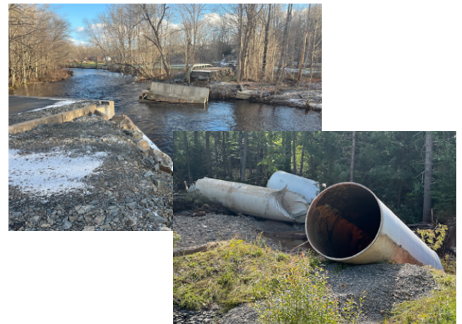
Flood damage near SCO
