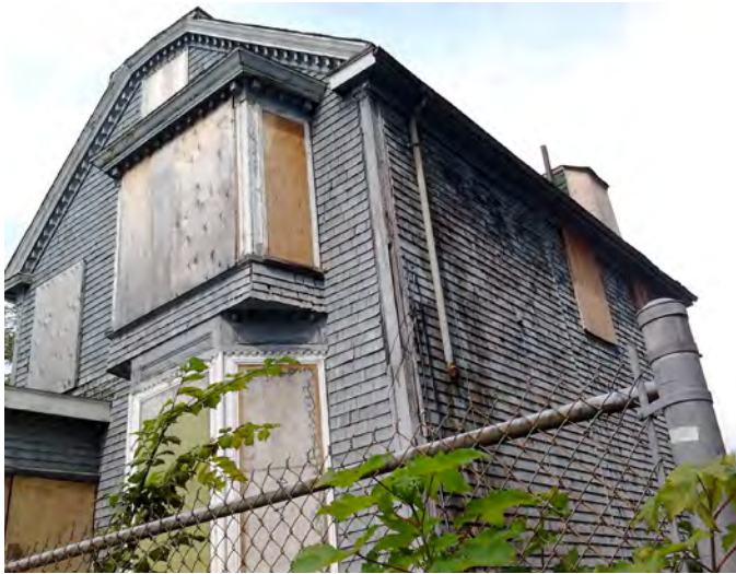
Figure 3 — Morris Office I. This and the following figures illustrate the range of sites available in a single geographic area, in this case Halifax. This building is associated with the Morris dynasty of Surveyors General of Nova Scotia (ca. 1749–1851), and is possibly the oldest extant workplace for applied astronomy in the country. This image shows it at a temporary site in 2012 awaiting restoration. While the Morris Office is now at a more long-term site, this illustrates the case that some structures of astronomical importance may be in temporary locations, and this will be reflected in their ALC entries. In the key to category site icons this is a mathematical practioner’s premises (see Figure 2). Photograph R.A. Rosenfeld.
